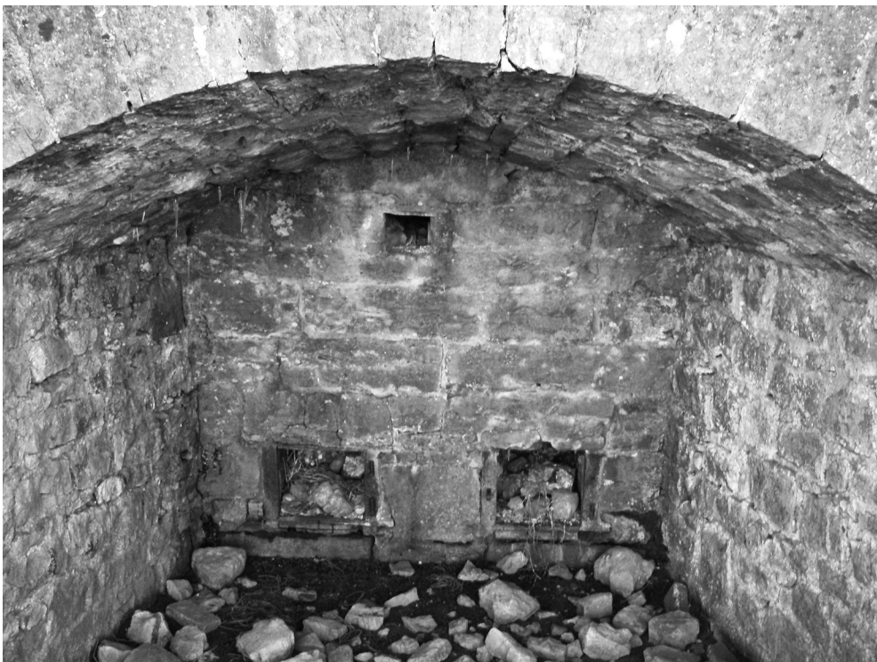
FIG. 8. A kiln with twin eyes, each with surviving framework for cast-iron doors, at Thrimby Out Scar.
